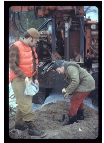
Water level meter in action in action; the MDSH chief soils engineer Don Malott, PE was reading water table.
